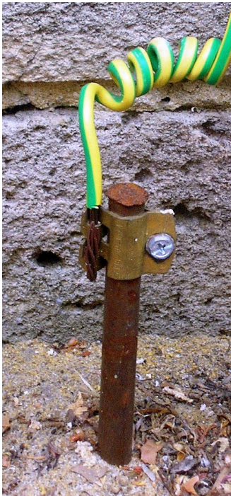
Earthing rod (typically solid copper or steel with copper outer layer) driven into the ground
